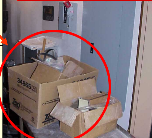
Improper Storage in front of Electrical Panel
